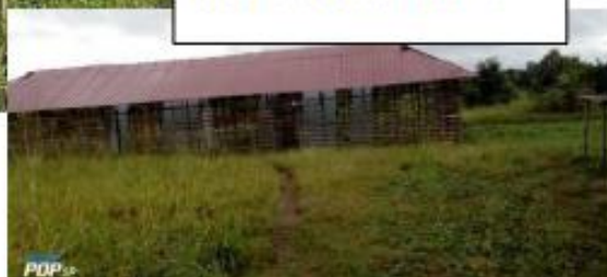
Before and after showing the progress of the renovation of the school on the outskirts of Yei.
